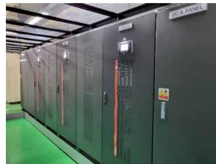
Adoption of high-efficiency Uninterruptible Power Supplies (UPS)
