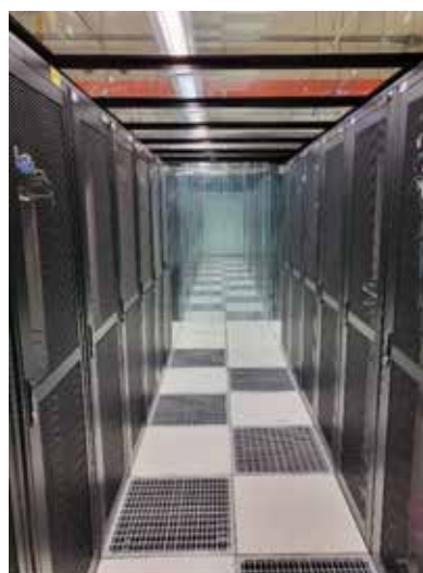
Hot/cold aisle configuration
